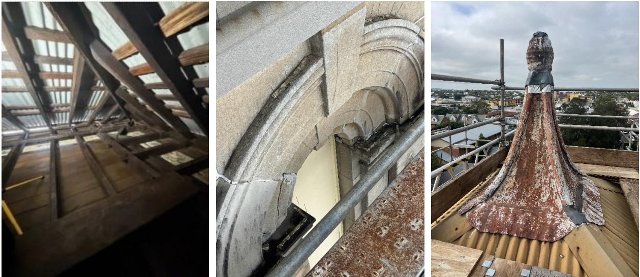
Images above: roof cavity after cleaning and repairs (left), damaged arched stonework identified for restoration (centre), the top of the tower which will also be restored (right).
