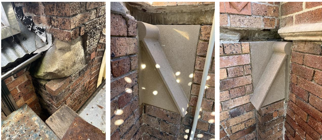
Images above: before stonework restoration (left), after stonework restoration of Building B (centre and right)
